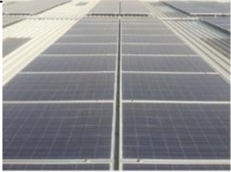
Solar Panels @ supplier site, Dharwad
