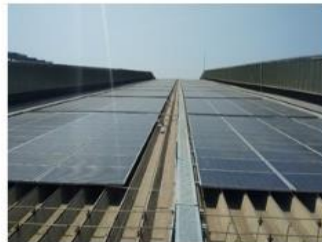
Roof top solar @ supplier site, Pune
