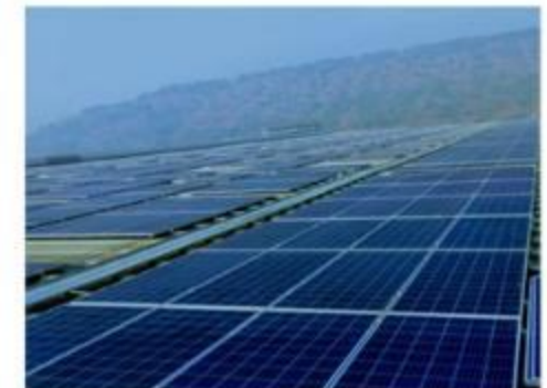
Roof top solar @ supplier site, Pune
