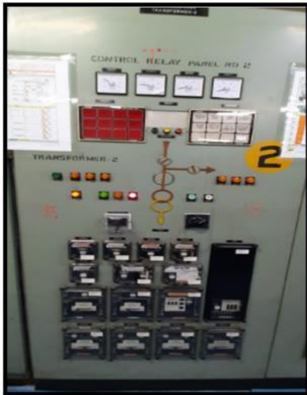
OLD CRP PANEL
