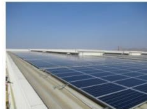
Roof top solar @ supplier site, Bangalore
