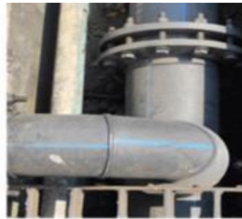
CONNECTED TO MAIN PIPE
