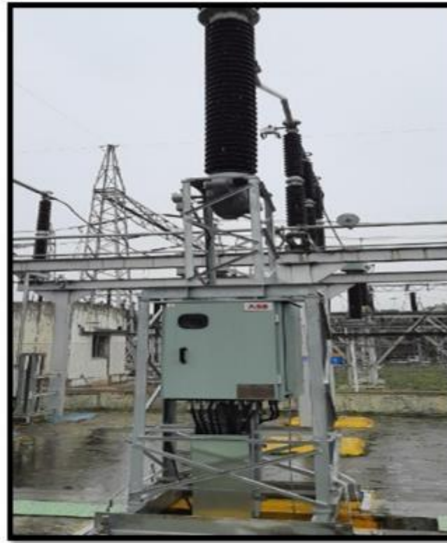
ELECTRICAL OPERATED BREAKERS
