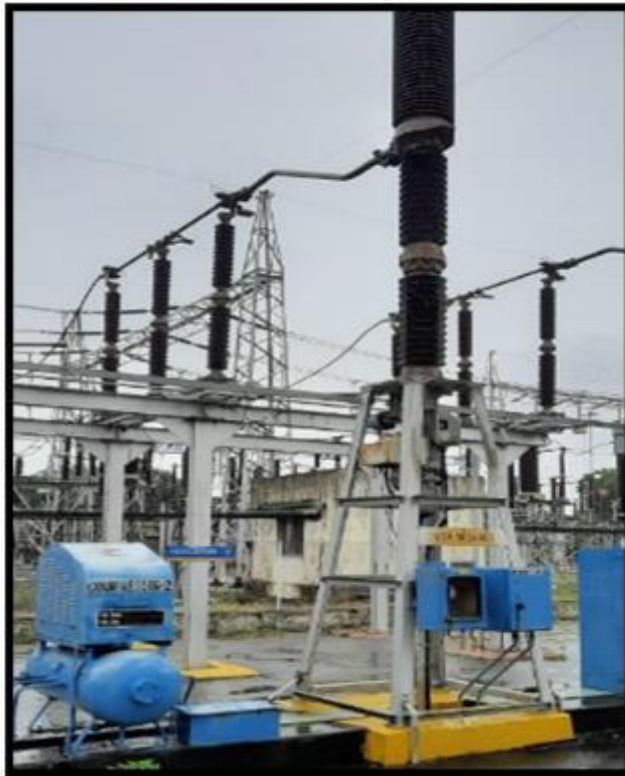
PNEUMATIC OPERATED BREAKERS
